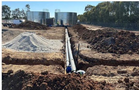
Moama Waste Management Facility fire system ring main installation to hydrants and newly installed fire water storage tanks and pump set in background.
